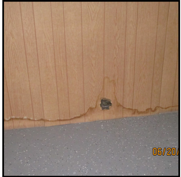
Water damage near sump pump in basement
