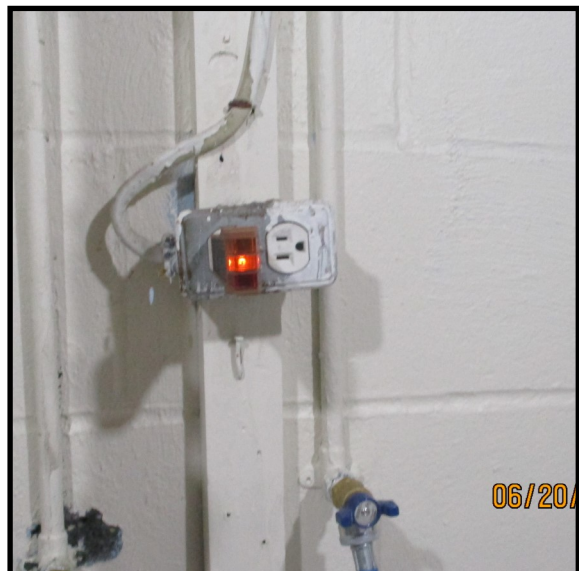
This outlet should be replaced with GFCI outlet
