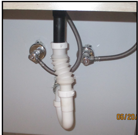
P-Trap underneath sink in 2nd bathroom
