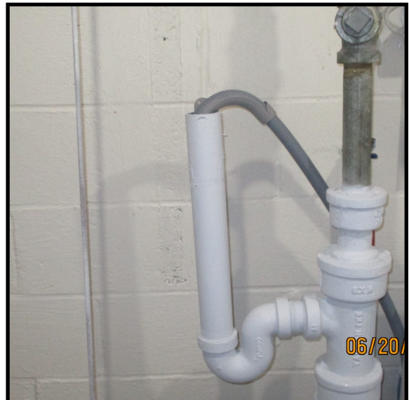
Discharge stuck from washing machine in laundry room
