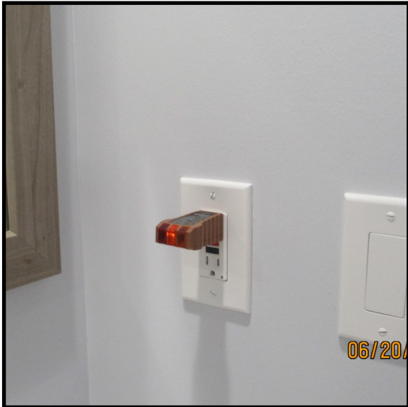
GFCI outlet in bathroom has no ground
