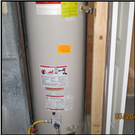
Old water heater
