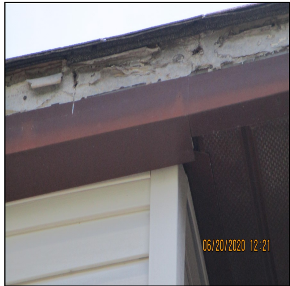
Peeling paint on roof fascia at the back of the house
