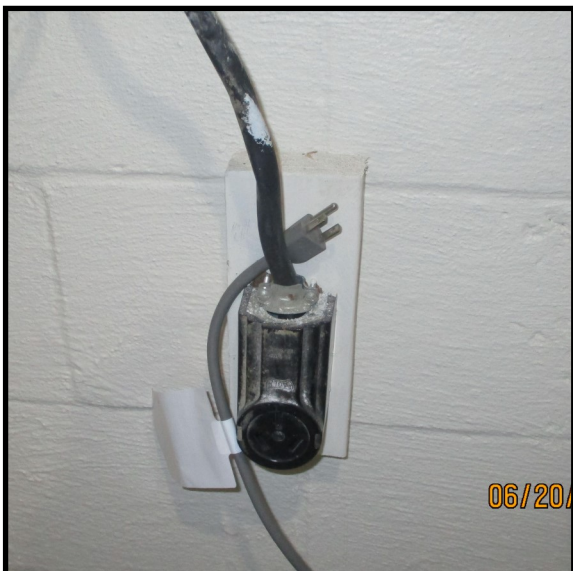
220 V outlet in laundry room
