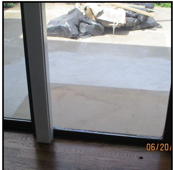
Broken patio entry sliding door in kitchen
