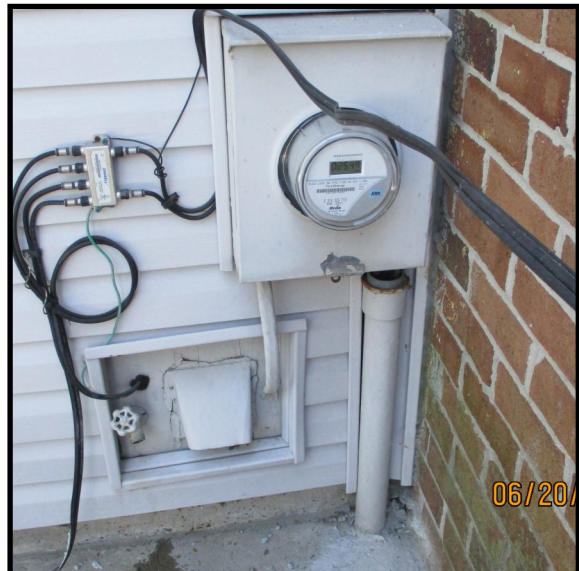
Electric meter located at the back of the house
