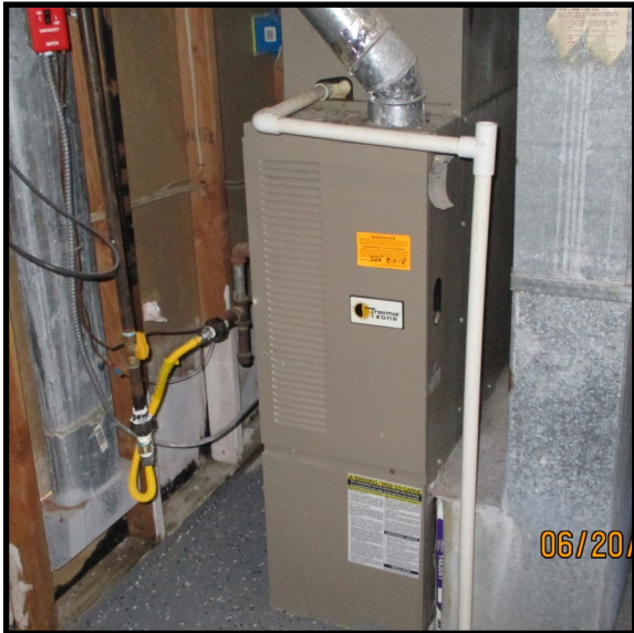
Broken gas furnace
