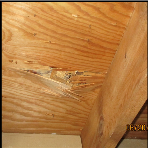
Damaged sub-flooring in basement
