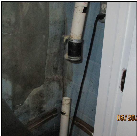
Discharge pipe is disconnected from sump pump
