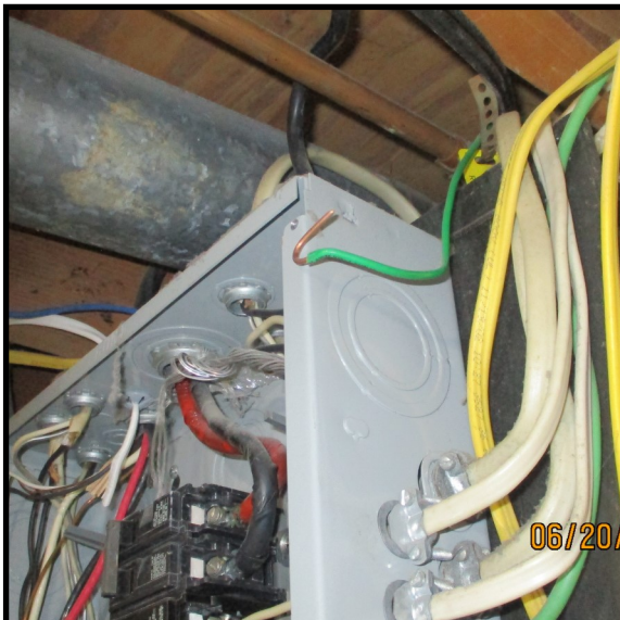
Ground wire is disconnected from main electric panel
