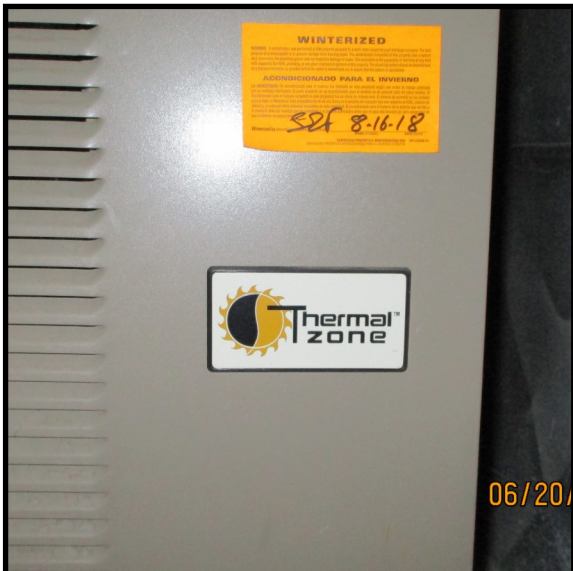
Closeup of furnace
