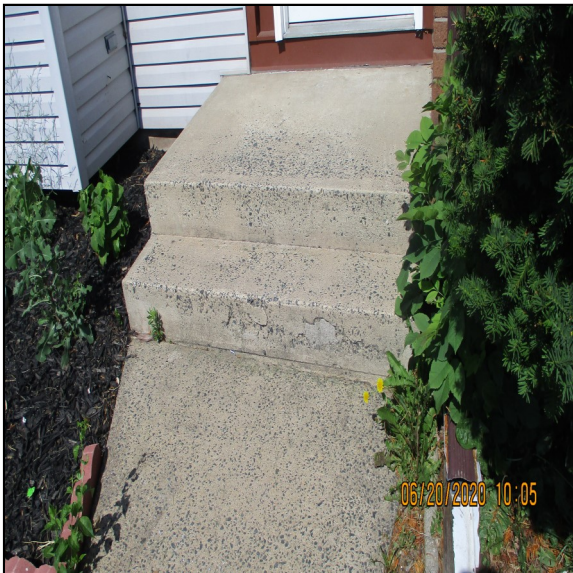
Front sidewalk and stairs. Step should be repaired.
