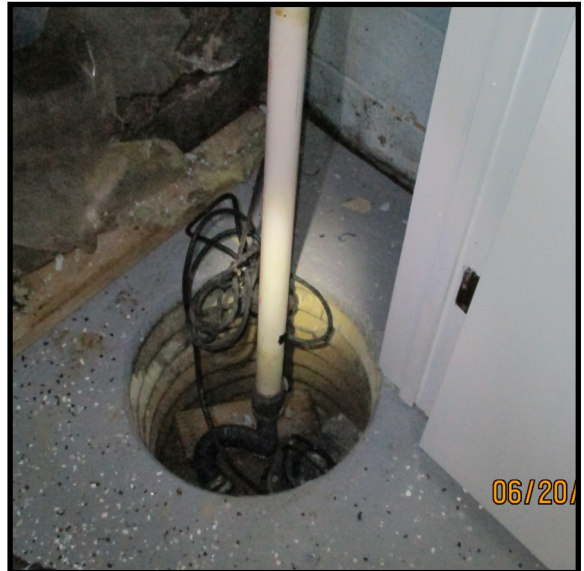
Sump pump in basement
