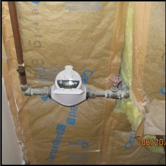
Water meter at the front of the basement
