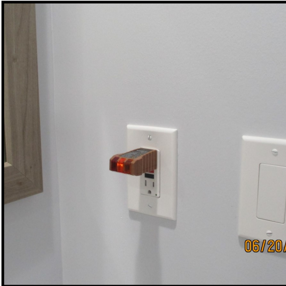
GFCI outlet in bathroom has no ground
